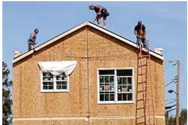
Ashley Custom Homes began assembling prefabricated homes in Baltimore City's Morrell Park neighborhood yesterday.
